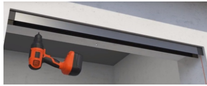
2 - Attach Top Guide to the Ceiling, with suitable SS fasteners. Pack if necessary; must be no greater than 10mm out of parallel to floor.
