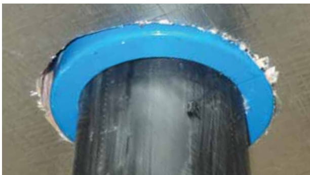
Figure 7 Penetration example - Kingspan Kooltherm® K10G2 Soffit Board installed tight around the fire collar and HDPE service pipe.
