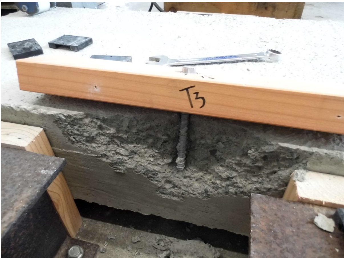
Figure 7. Out-of-plane shear, typical slab edge breakout failure.
