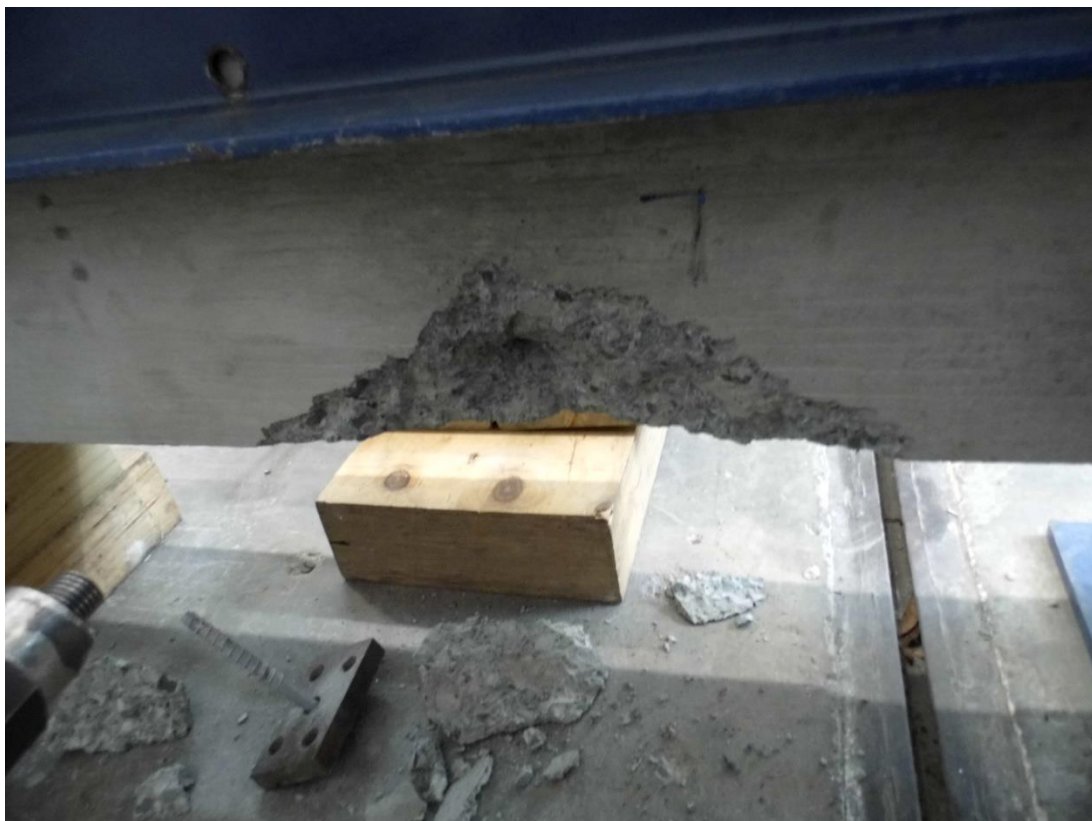
Figure 9. Tension, typical concrete breakout failure.
