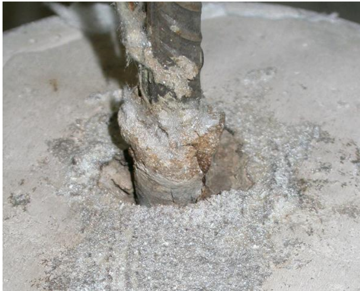
Figure 9: Bond failure after fire exposure
