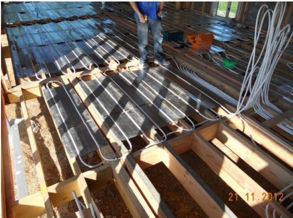
Spreader plate installation with joists at ground floor close to ground level
