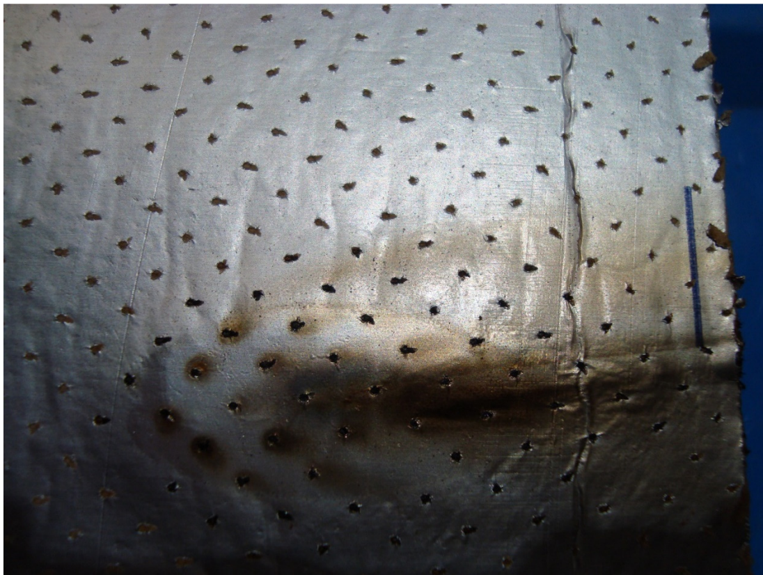
Discoloration of metallic facing material due to needle flame
