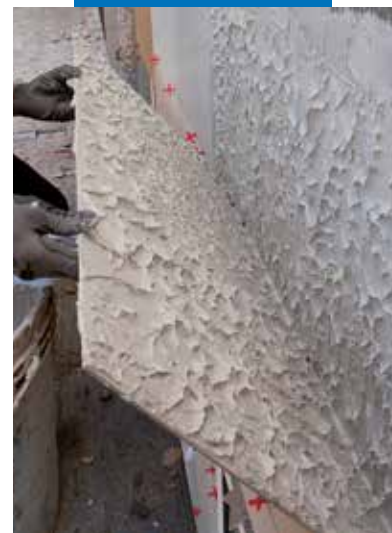
Checking the back face of the tile if it is completely buttered when laying on an external façade
