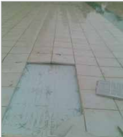
Fig. 5.1 - Tiles detached from a substrate due to compressive stresses
