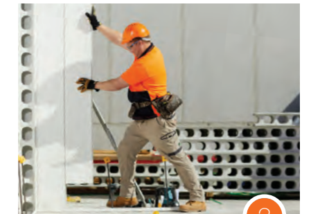
3 And simply slide down to seat into the floor tracking and form a wall
