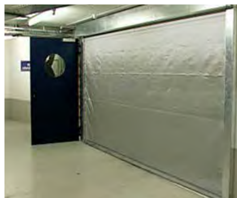
Fire and smoke compartmentation in a basement carpark with additional egress door. An egress door prevents occupants from driving out of the car park and blocking fire fighting activities
