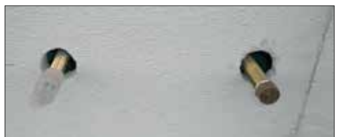
Fig. 3.3 – Neat finishes of installed services
