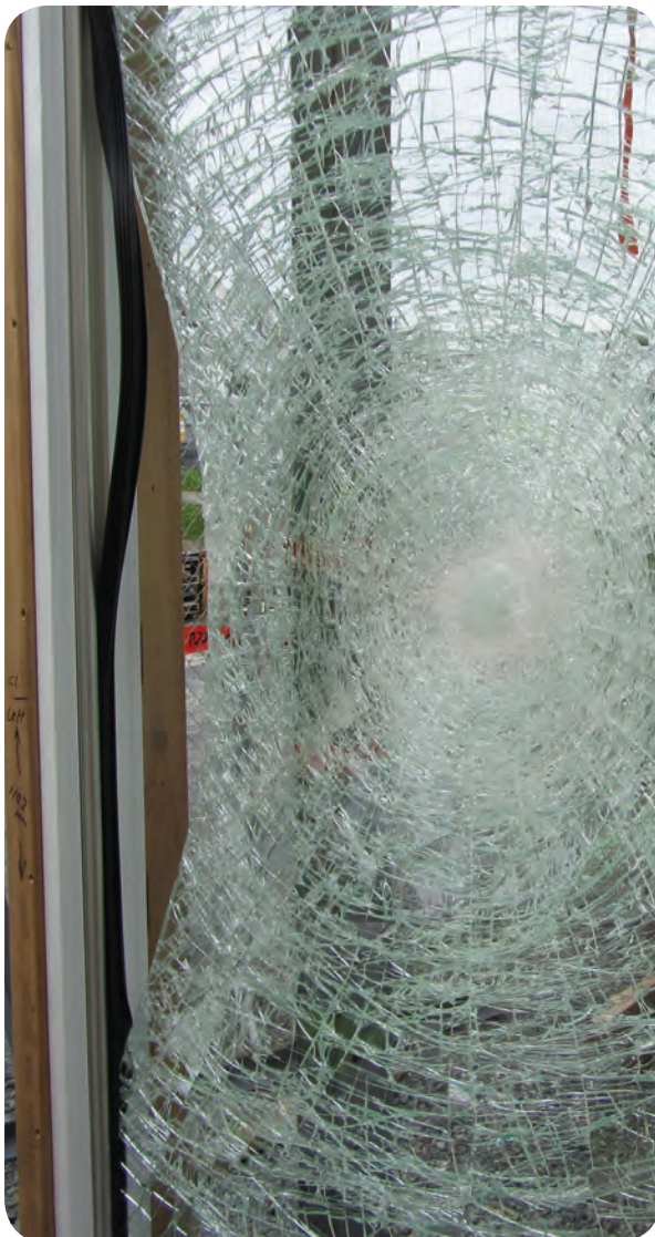
Window System Failure
