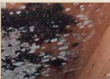
Fig. 3. Mould in the building structure
