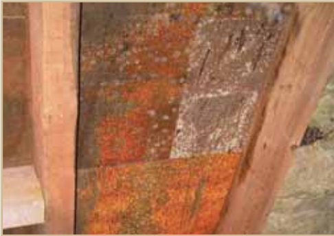
Fig. 44. Mould in the building envelope
