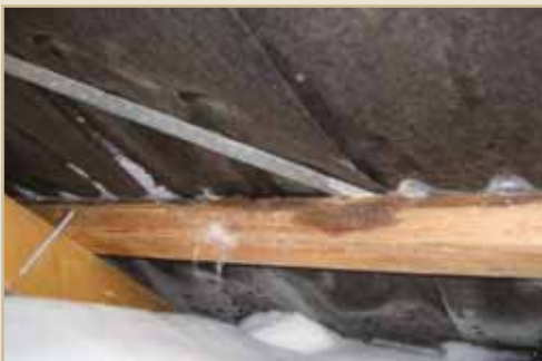
Fig. 49. Condensation on the roof underlay due to poor airtightness
