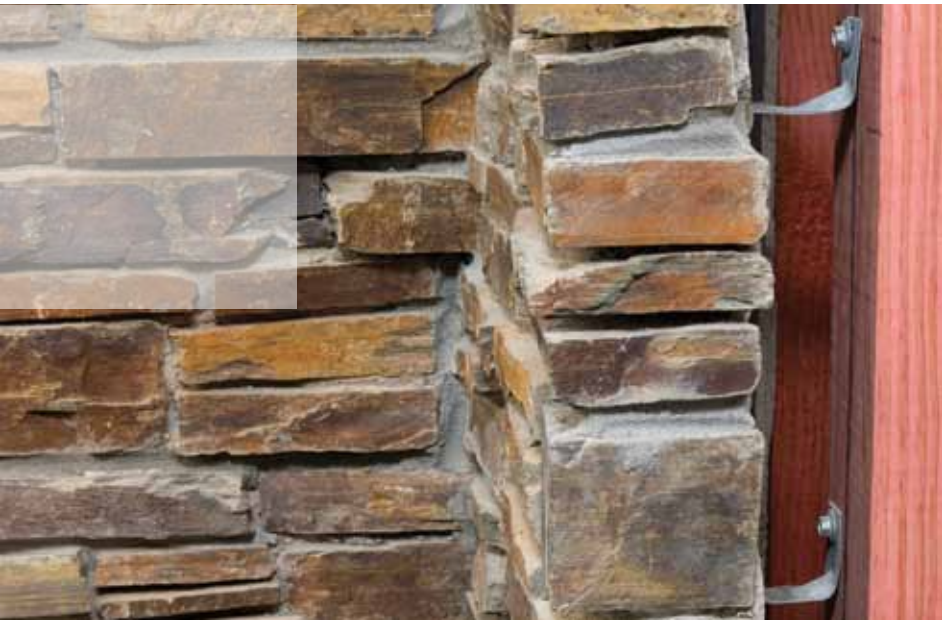
Autumn Horizon showing the use of brick ties to create a drained and ventilated cavity
