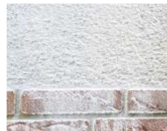
Washed off facade without QS technology
