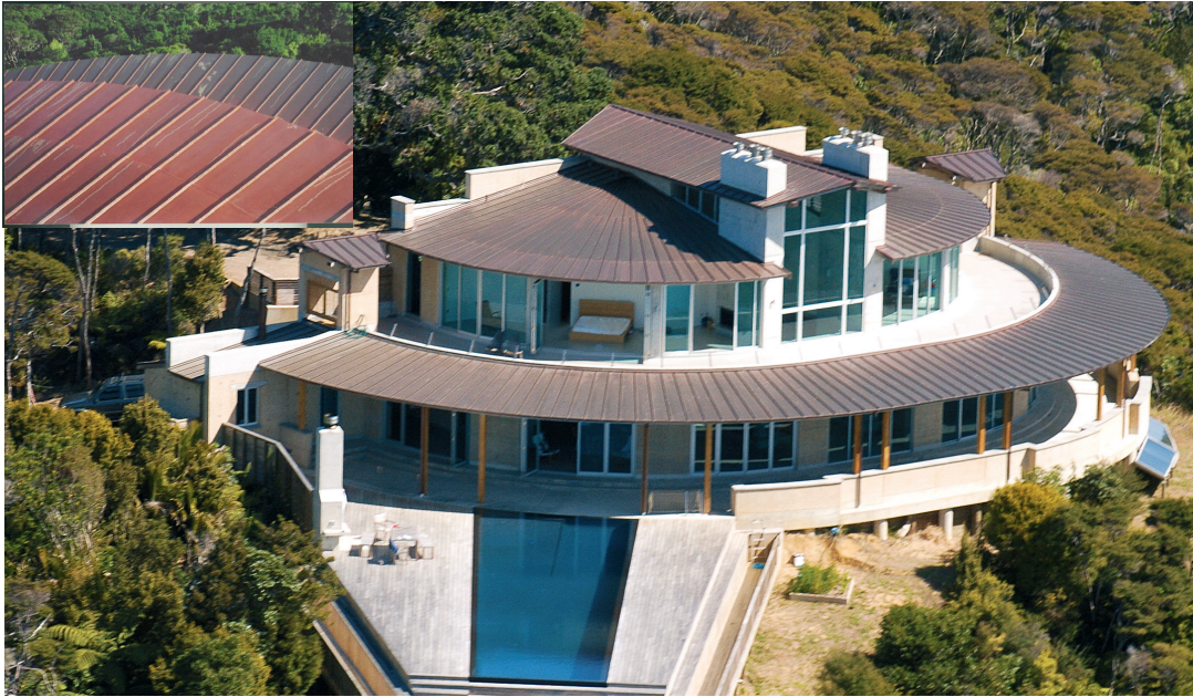
smart tray™ custom panel splayed sheets form this curved roof feature - copper
