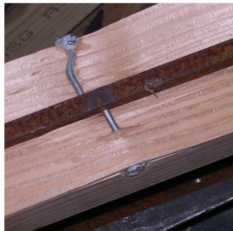
Figure 2. Poor penetration of pins
