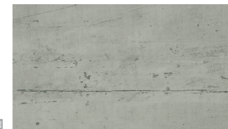
2585 Cold Cracked Concrete 177.8 x 1219.2mm
