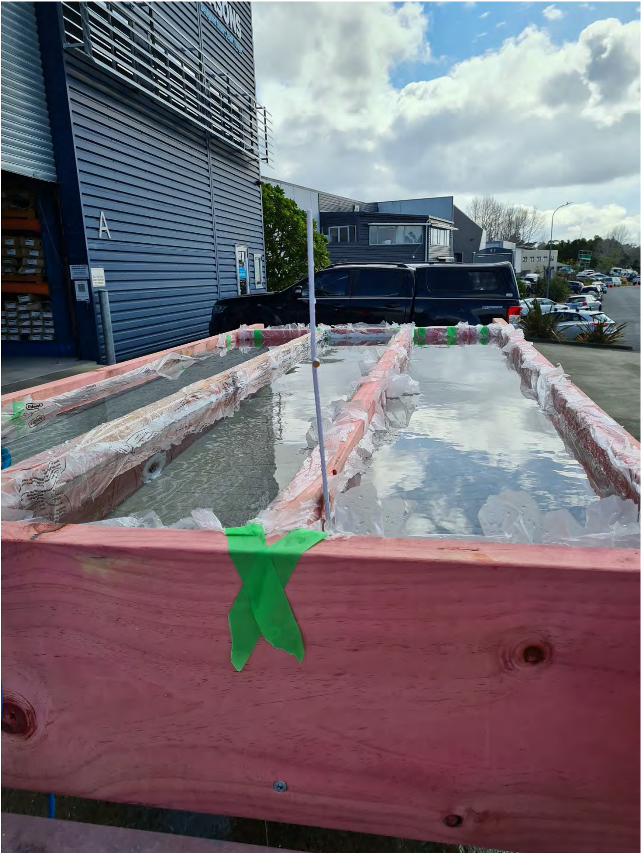
Photo 2: Water holding at minimum specified time (15 minutes) prior to failure
