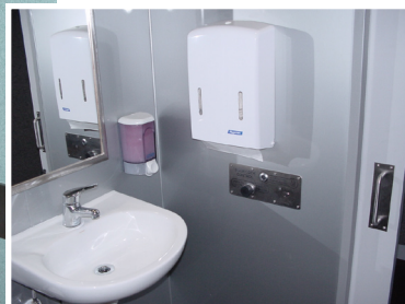
▶ Inside view of toilet; heavy duty push button and indicator panel (below paper towel dispenser).
